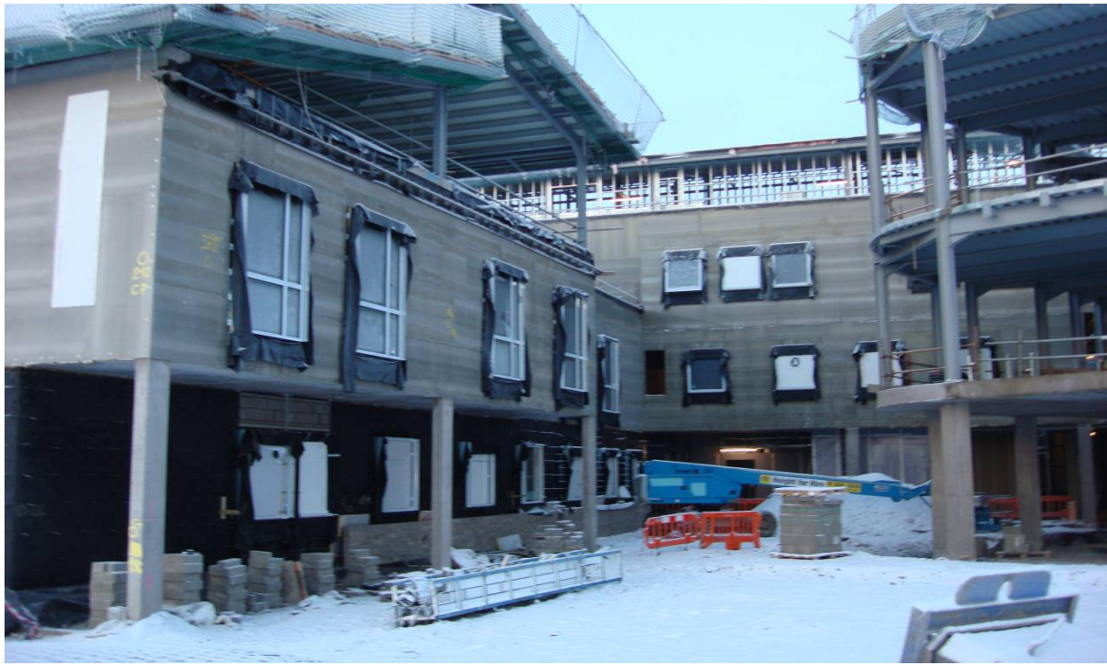
Photograph 3 – Block B windows. Inclement weather conditions (November 2010)
