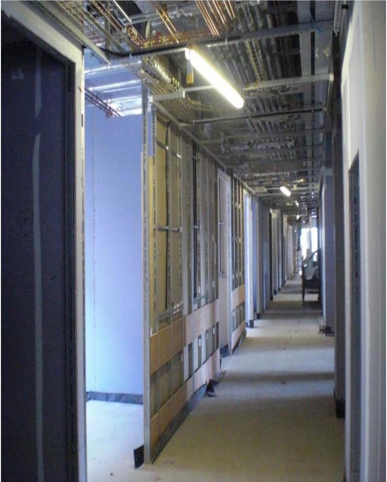
Photograph 8 - Block J – Interior Fitout – Indicating Progress of Plasterboard Partitions and M&E Installations
