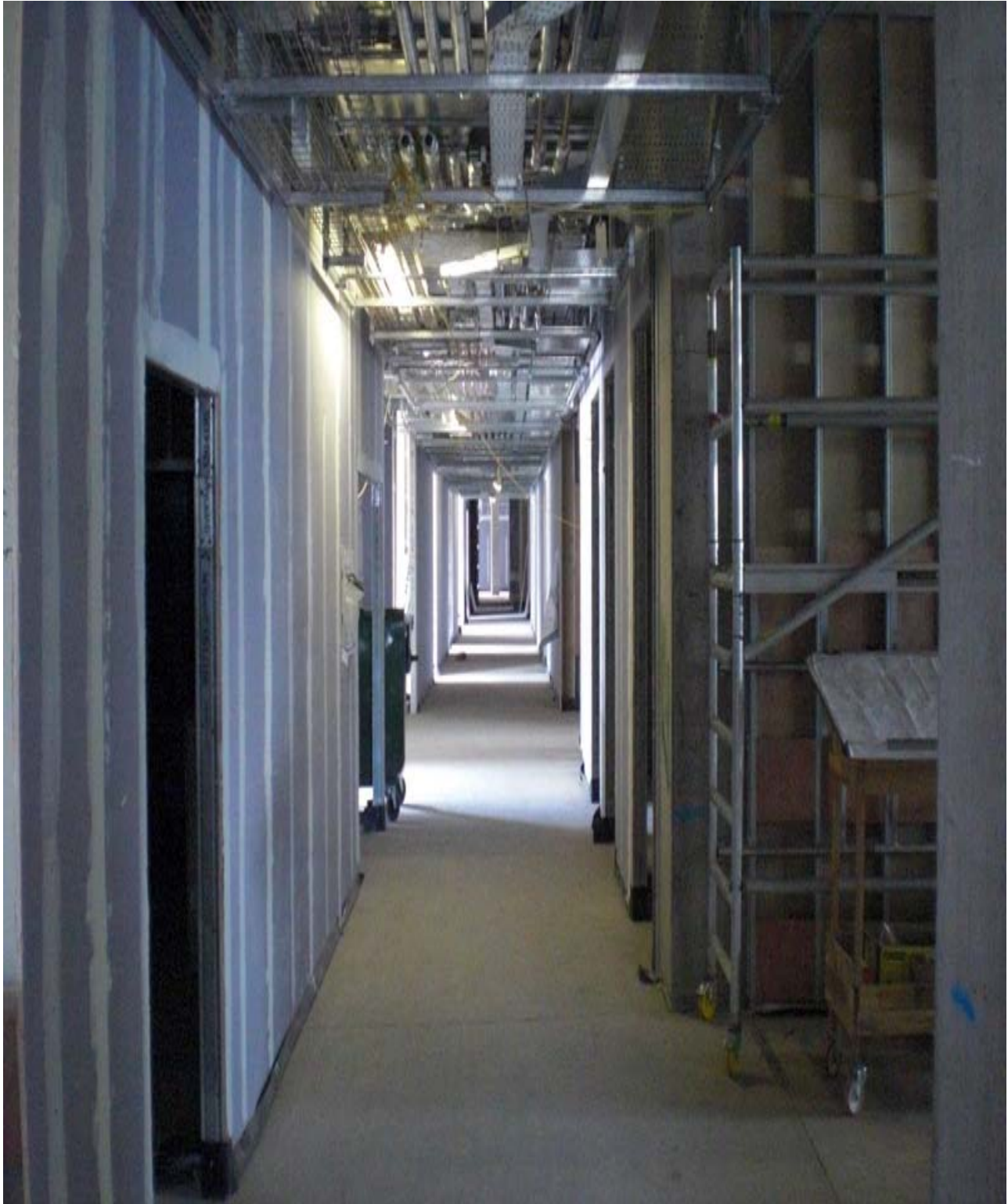
Photograph 9 - Block J – Interior Fitout – Indicating Progress of Plasterboard Partitions and M&E Installations
