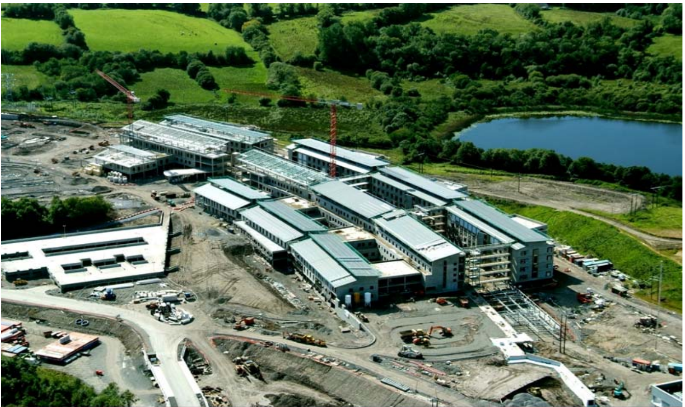
Photograph 4 – North Elevation Overview From Energy Centre
