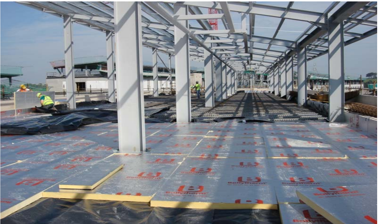
Photograph 6 – Plantroom – Block B1. Isolation works previous screed will be poured on the plantroom in Block B
