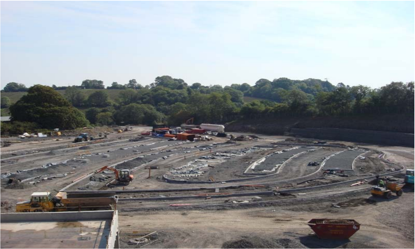
Photograph 9 – South Car Park – External Works Progressing on the gabion walls complete for that area
